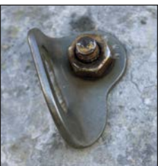
Corroded Rocklands bolt - DANGEROUS!
